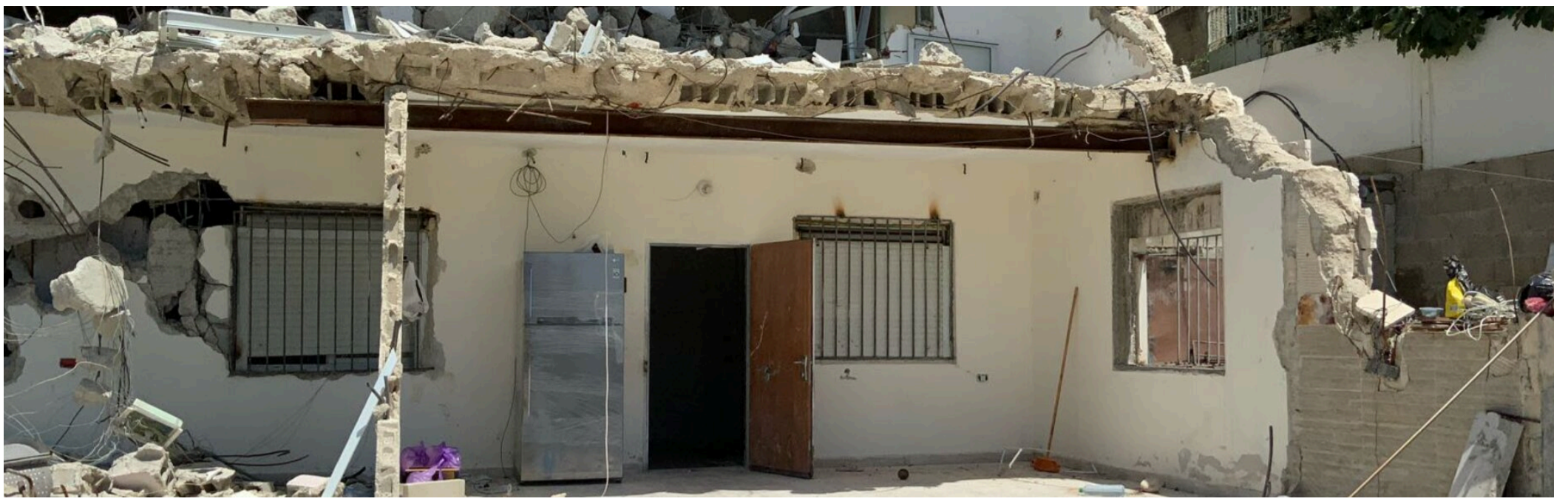
This was the home of a family in the Ras al 'Amud area of East Jerusalem. The family was forced to demolish it following orders by Israeli authorities citing lack of a building permit, which is rarely granted for Palestinians. Photo by OCHA
