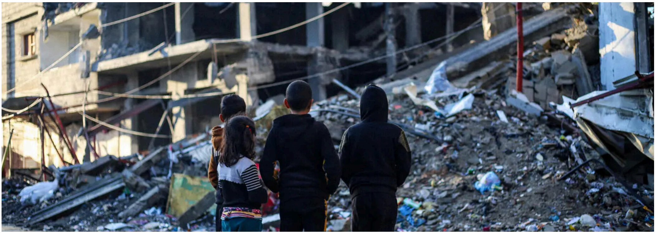
Children stand in front of a house demolished by a bombardment in the city of Rafah, south of the Gaza Strip. Photo: UNICEF/Eyad El Baba
