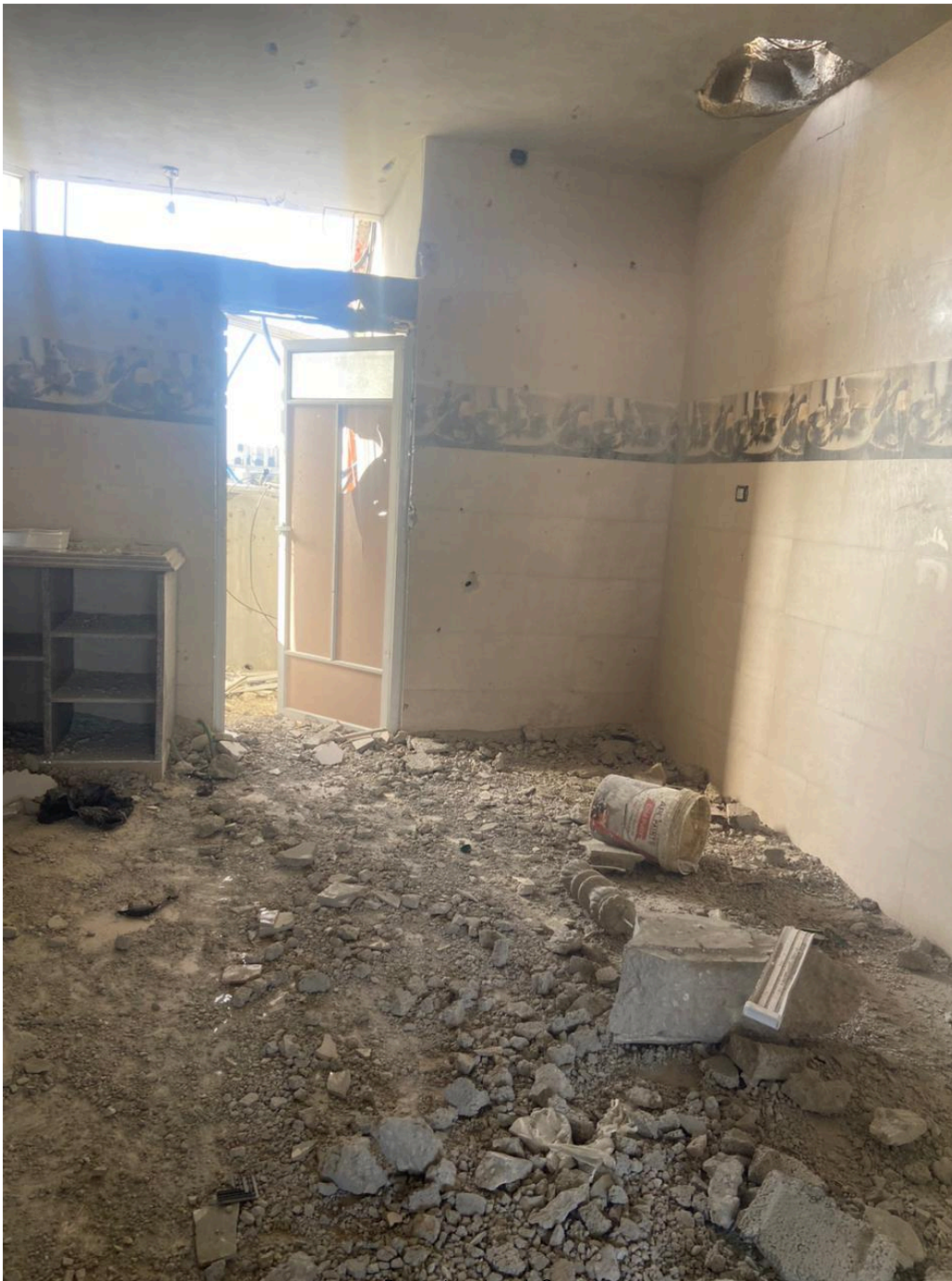
Damage to my home in Gaza.
